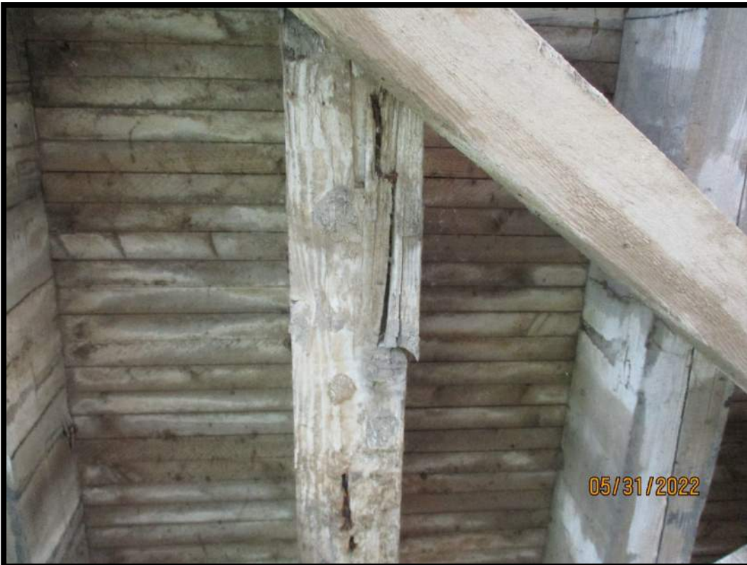
Figure 30: Some splitting noted in timber stringers
