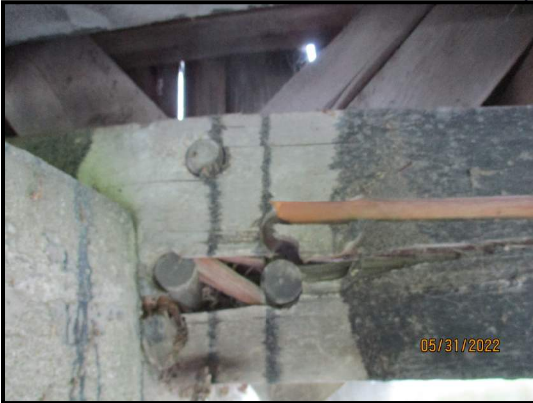
Figure 17: Truss Bearing at Pier – NW Corner – Lower chord failed, connection pins displaced
