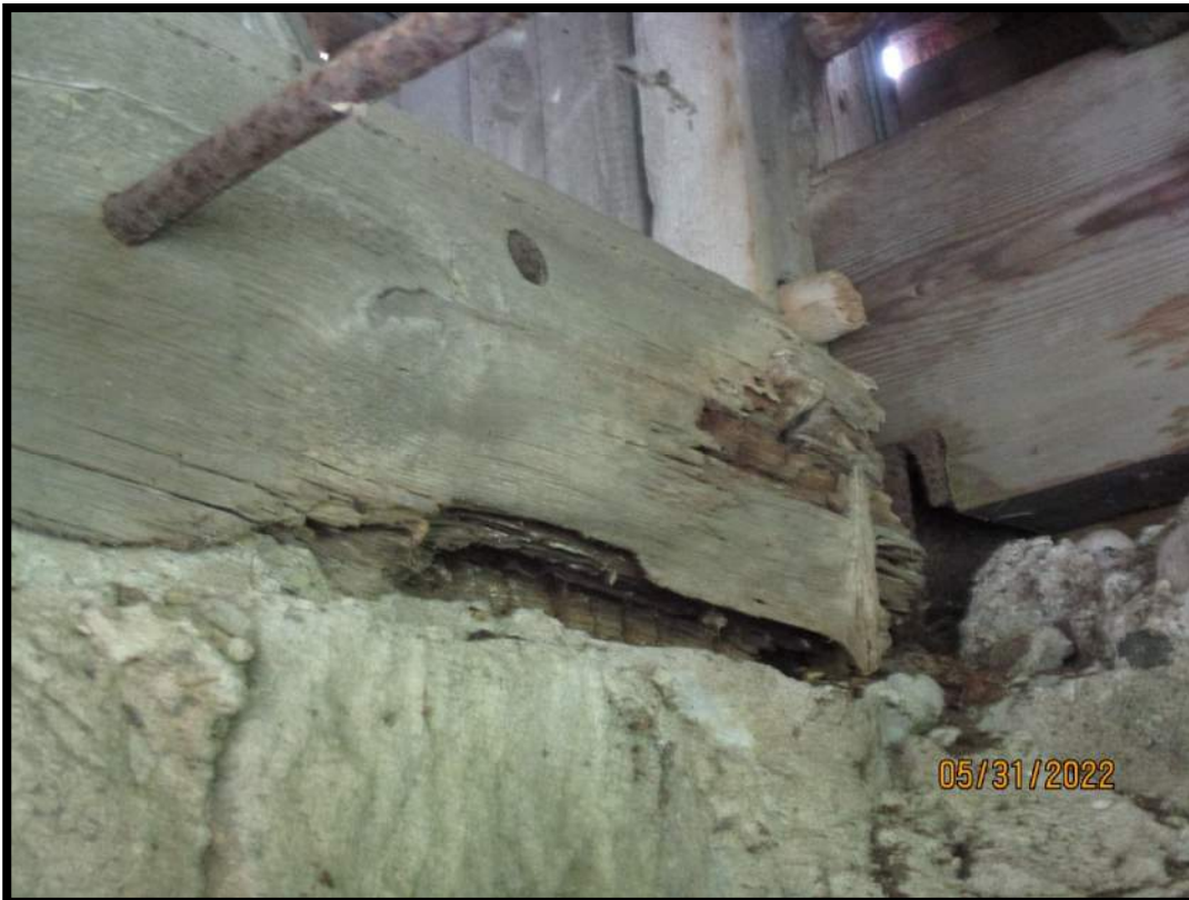
Figure 22: Truss Bearing at Abutment – NW Corner – Significant section loss to timber
