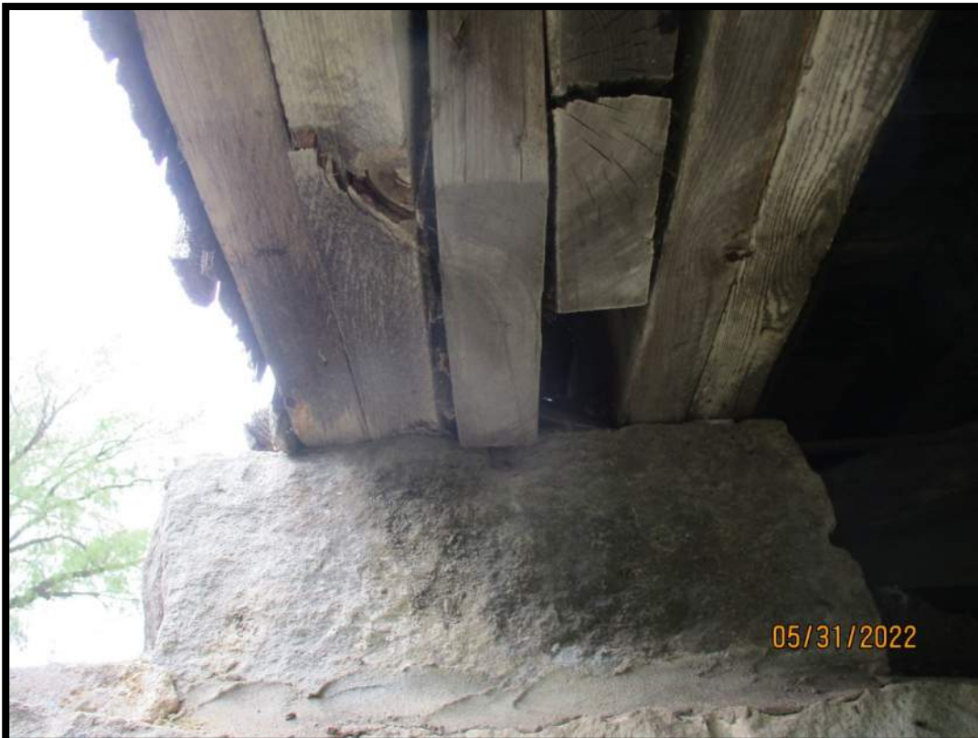
Figure 24: Truss Bearing at Abutment – NW Corner – Lower chord lamination split and web member split
