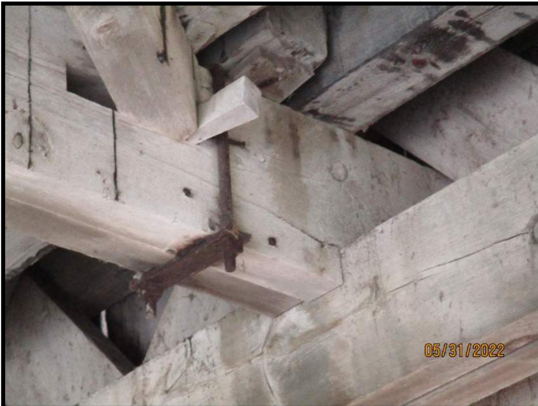
Figure 26: Floor Beam Near South End of Deck – Split originating from notch, previously repaired with steel clamp
