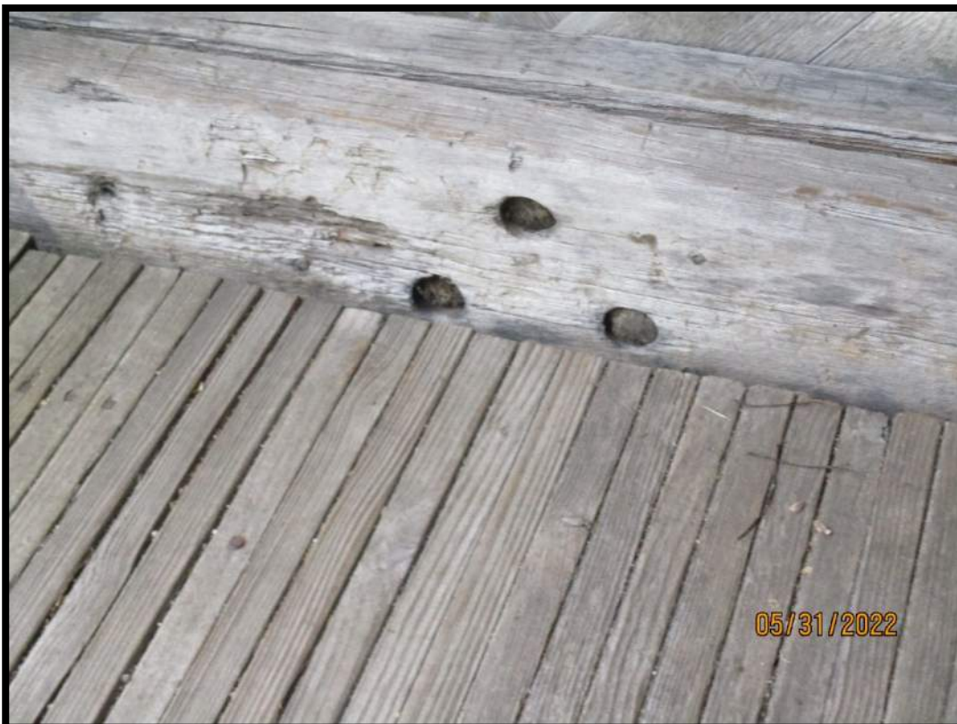
Figure 10: Truss connection pins rotting
