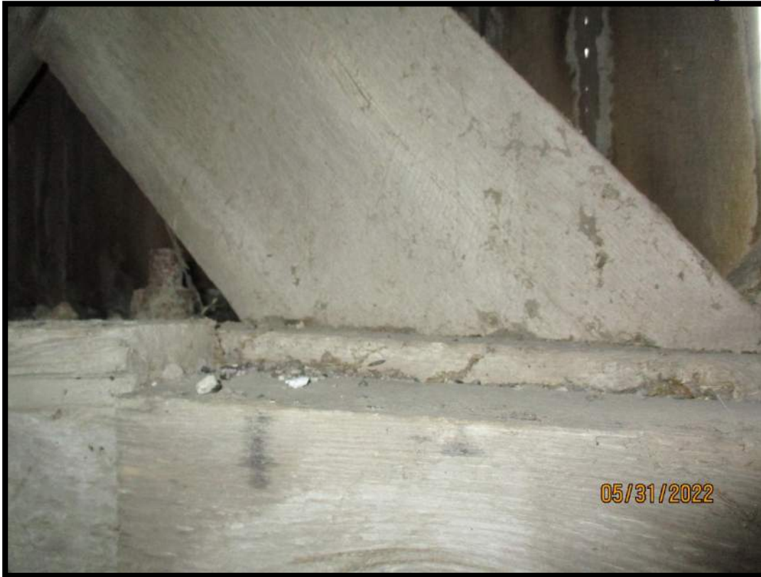
Figure 11: Truss Bearing at Pier – SE Corner – Interior lamination has dropped +/-1"
