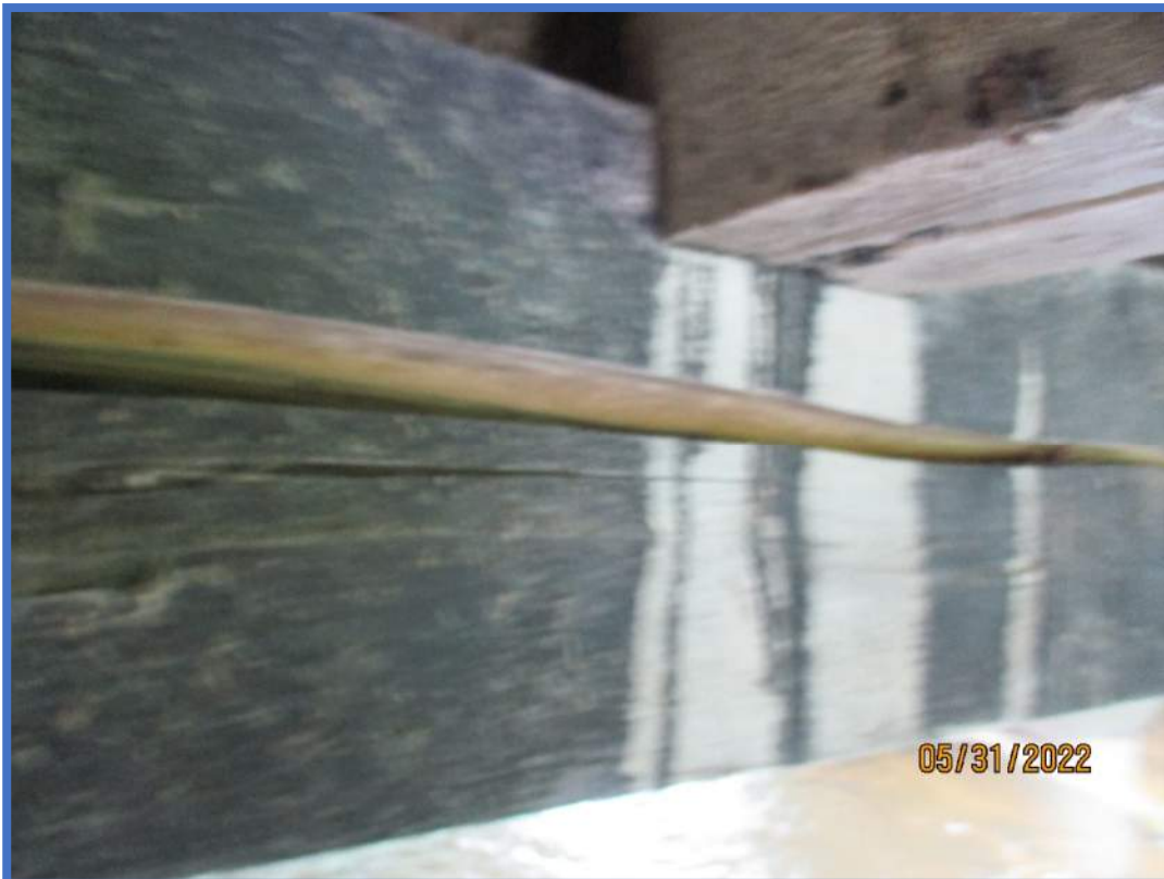
Figure 18: Truss Bearing at Pier – NW Corner – Crack opens 3" and extends past floor beam
