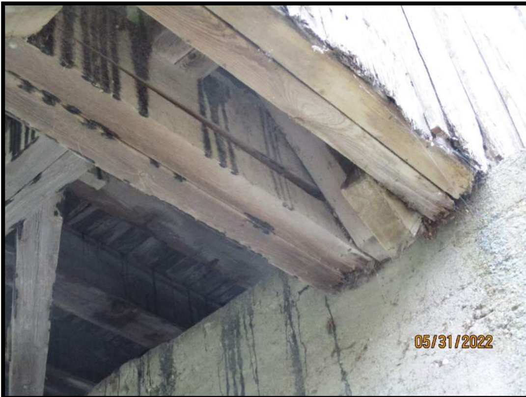
Figure 20: Truss Bearing at Pier – NW Corner – Interior laminations split and dropped
