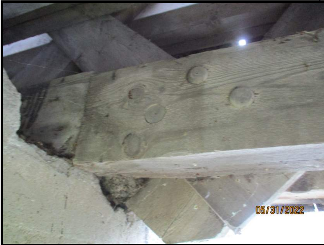
Figure 13: Truss Bearing at Pier – SE Corner – Interior lamination has dropped +/-1"
