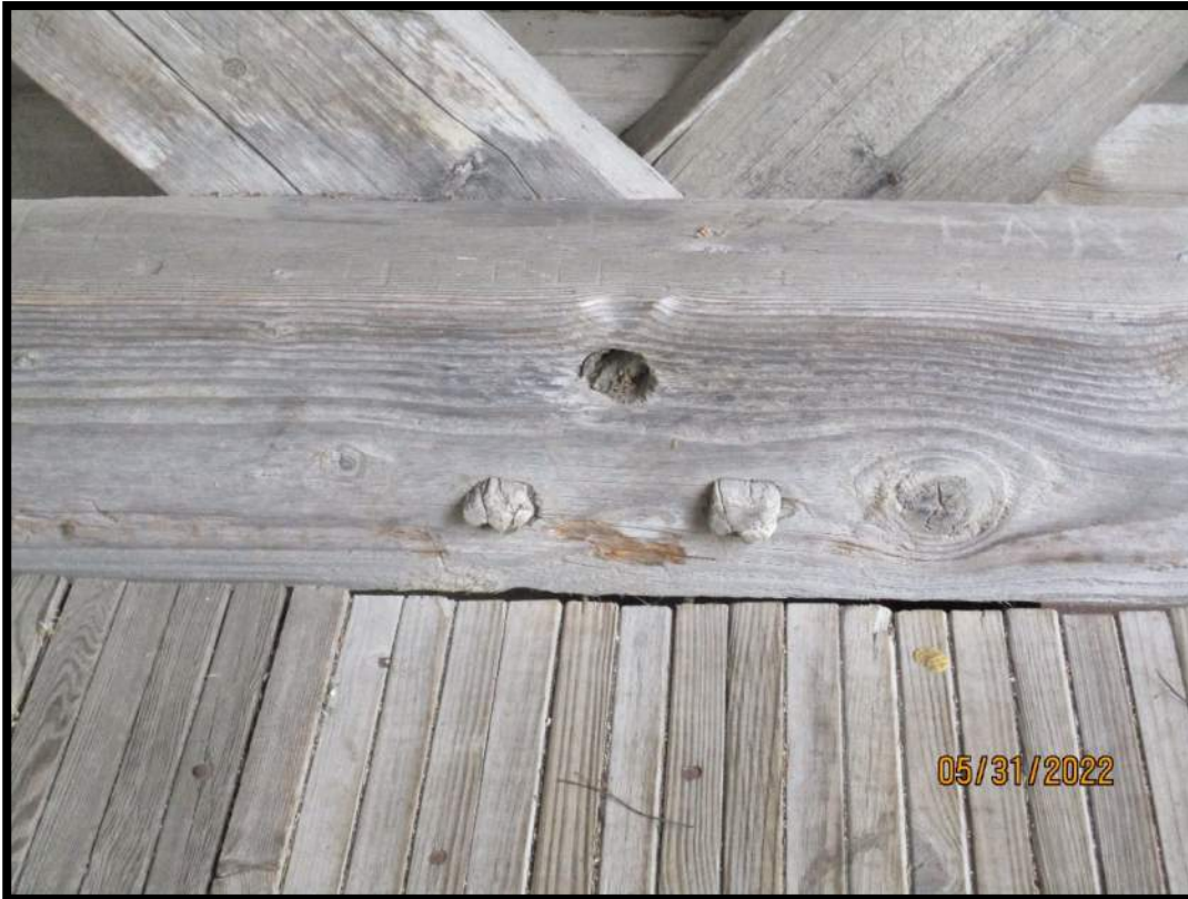
Figure 9: Truss connection pins rotting
