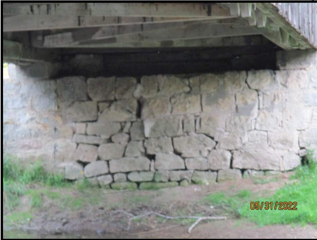
Figure 31: Loss of mortar at masonry abutment
