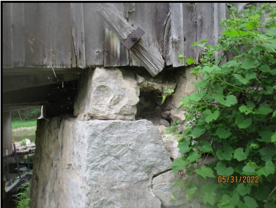
Figure 28: NE Corner of abutment – Loss of stone and mortar
