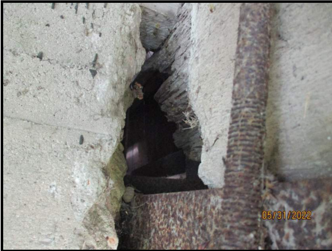
Figure 7: Truss Bearing at Abutment – SW Corner – 100% section loss of lower chord
