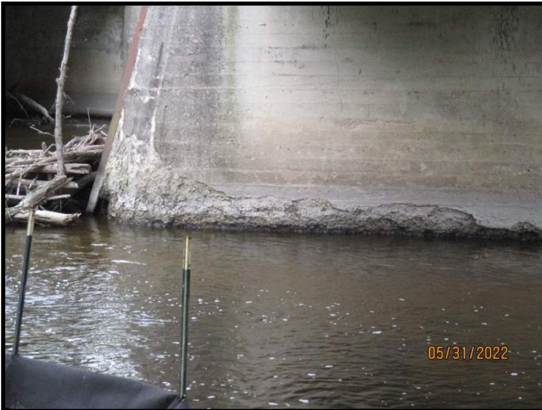
Figure 32: Spalling at base of concrete pier
