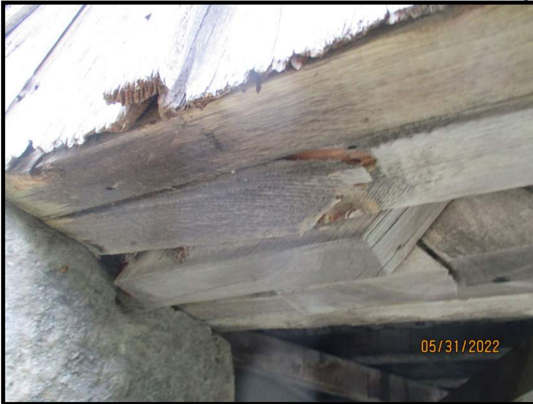
Figure 23: Truss Bearing at Abutment – NW Corner – Lower chord lamination split at bearing
