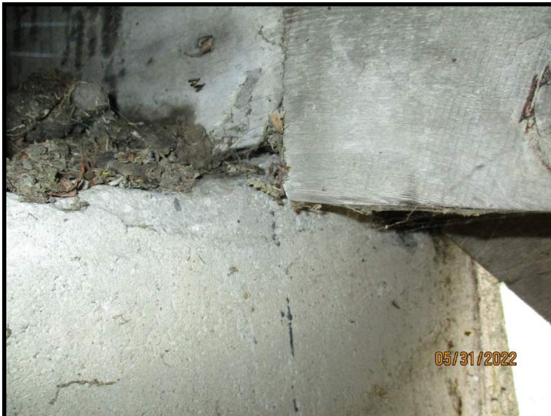
Figure 12: Truss Bearing at Pier – SE Corner – Interior lamination has dropped +/-1"
