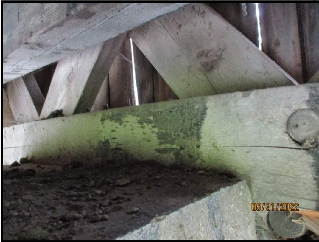
Figure 19: Truss Bearing at Pier – West Side – Truss is continuous, cracking on both sides of pier
