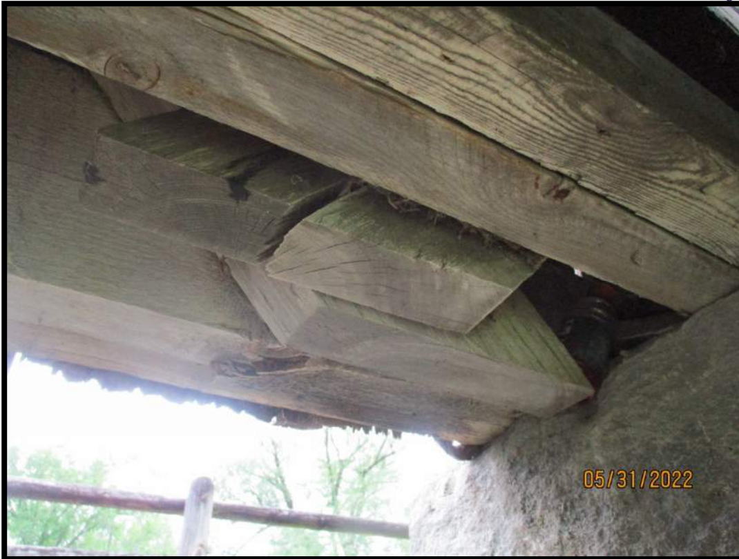
Figure 25: Truss Bearing at Abutment – NW Corner – Web member split
