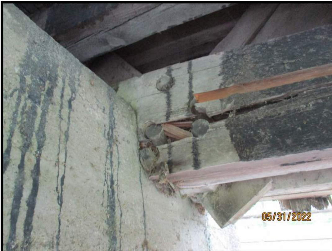
Figure 16: Truss Bearing at Pier – NW Corner – Lower chord failed, connection pins displaced
