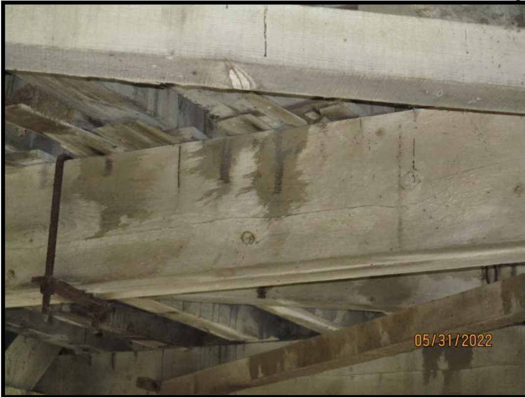
Figure 27: Floor Beam Near South End of Deck – Horizontal split continues full length
