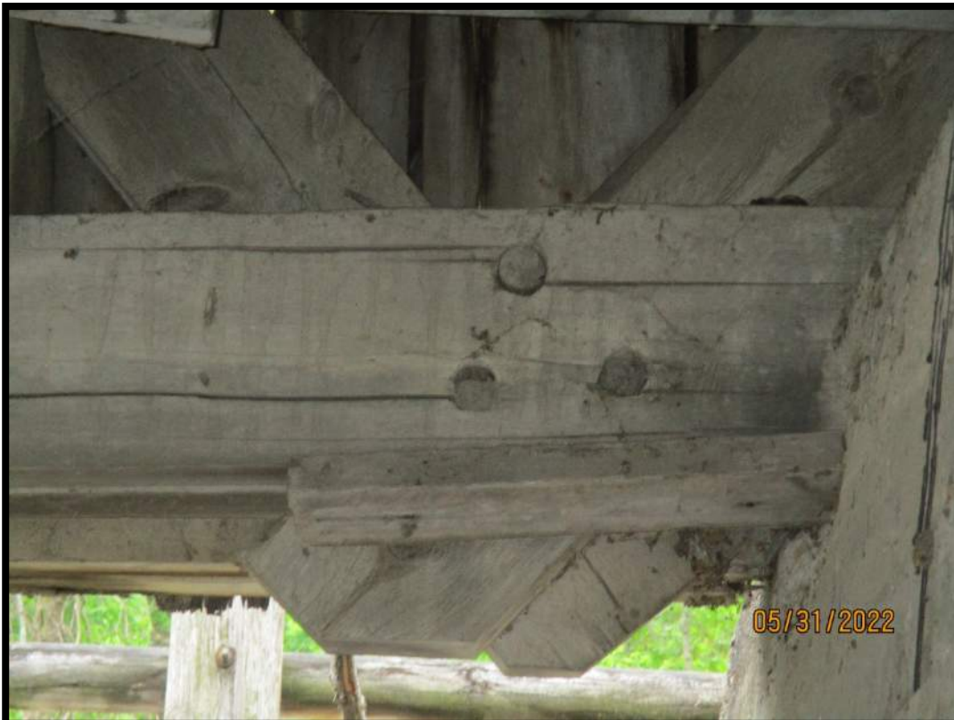
Figure 14: Truss Bearing at Pier – SW Corner – Splitting starting with interior section loss
