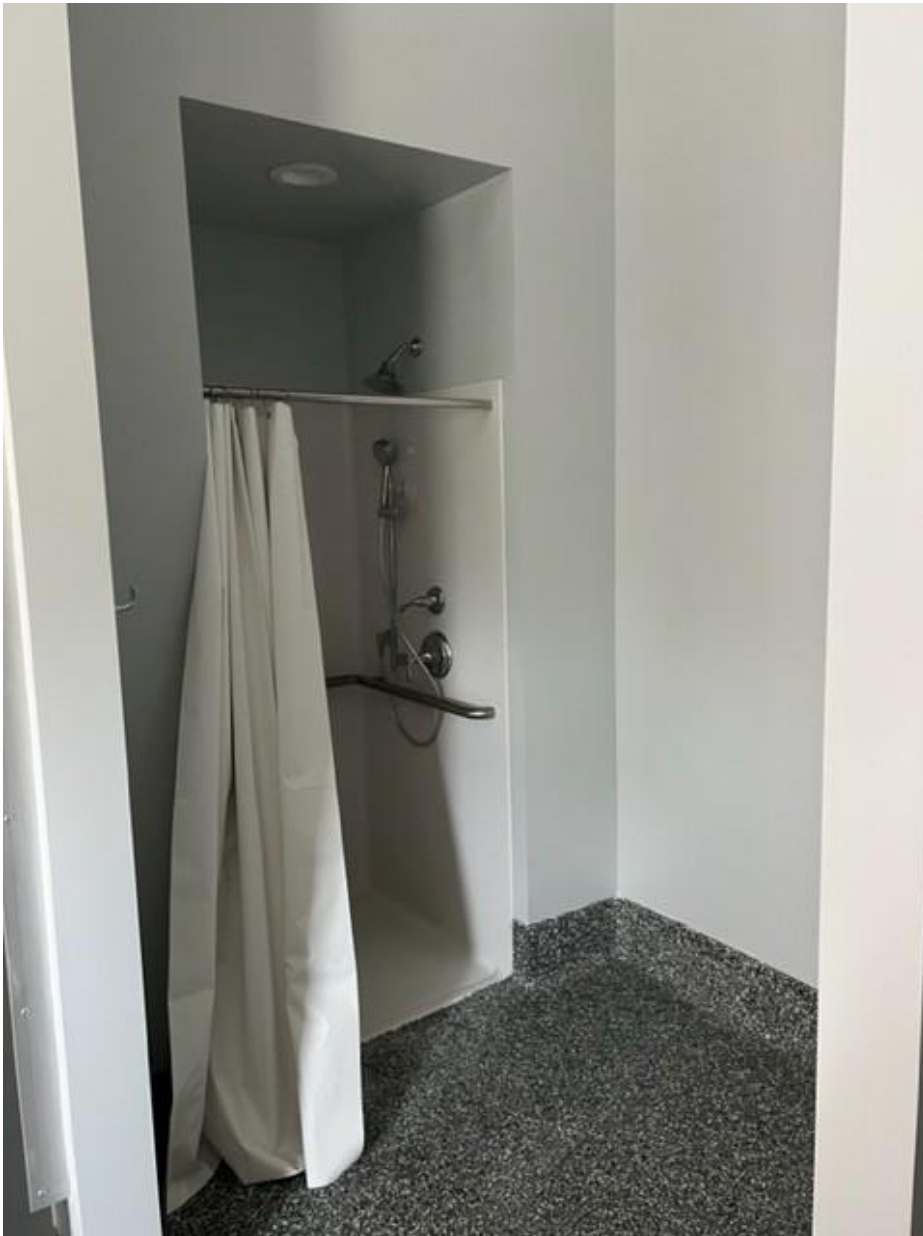
ADA compliant shower in Men's Bathroom at HH Peters Youth Camp
