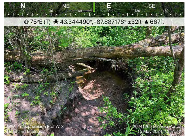
Photo #76 WW-2 steep erosion east of W-3
