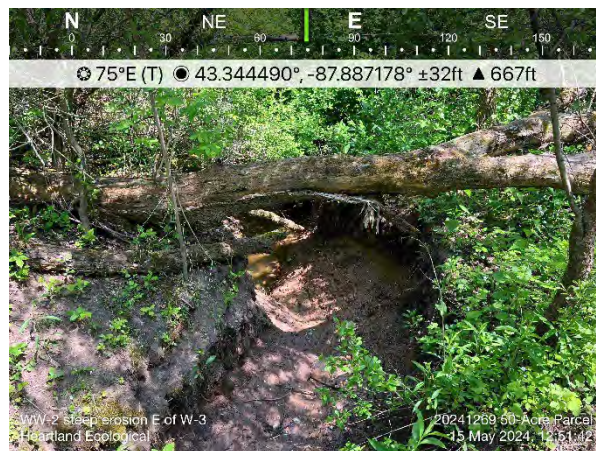
Photo #76 WW-2 steep erosion east of W-3
