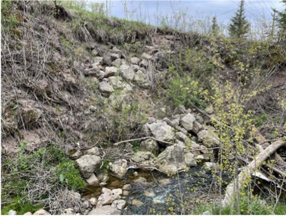
Photo 3: North bank erosion in Oakland Green Park. The City of Port Washington has historically dumped riprap and large stone on the banks.
