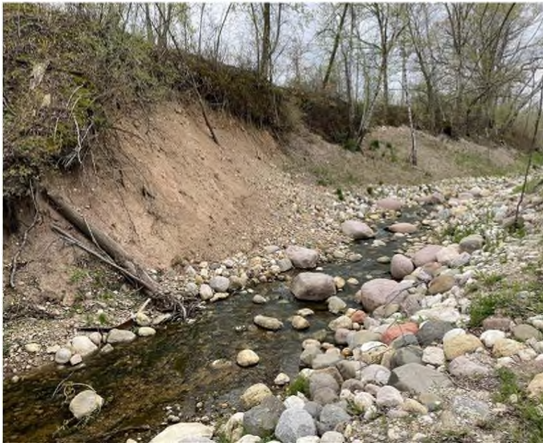
Photo: South bank erosion at the downstream portion of the restored channel.
